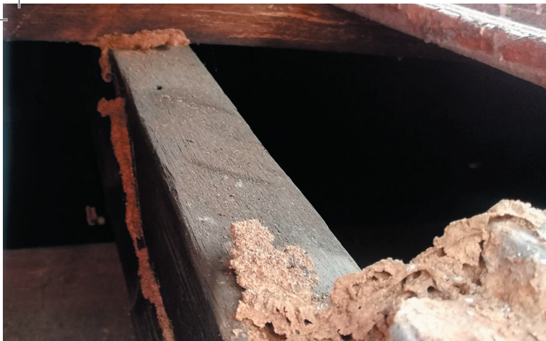
ABOVE Termite damage in the roof void of Chettiar Hall.
